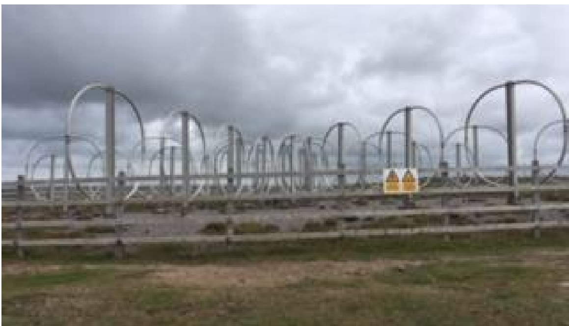
Figure 39: Penhale Camp telecommunications site on Penhale Point (credit LLCA Team)
